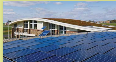
The Hanover Township Building features a green roof on the Administration Building and solar panels on the Public Works roof.
